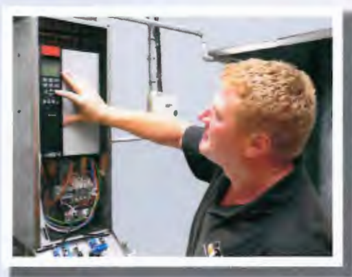
Verne is commissioning a 28 unit installation in NZ
